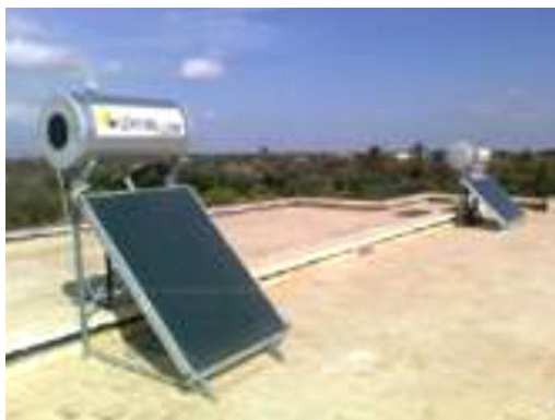
Figure 171: Solar water heaters installed on the rooftop of the Dar Amys Villa.
