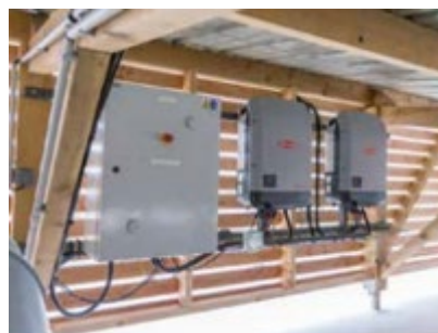
Figure 49: Solar inverter and sensors of the PV system
