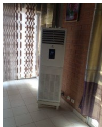
Figure 123 : Floor standing air conditioner have been installed in some rooms.
