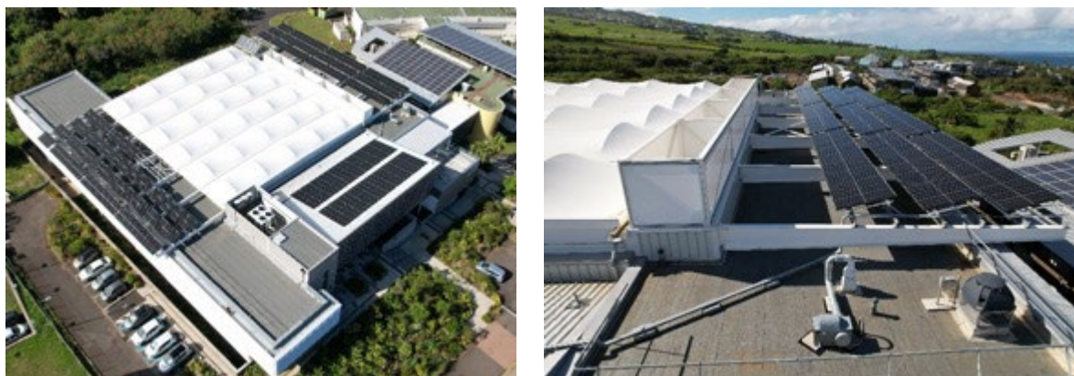
Figure 65: Solar thermal and PV panels have been installed on the rooftop of the building.
