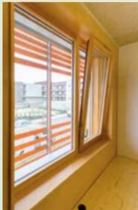
Tilt and turn windows used in Izuba energies building
