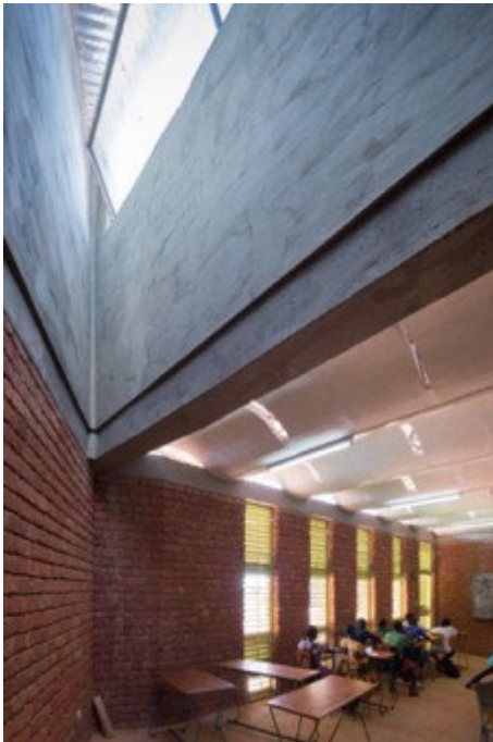
Figure 100: Interior view of the classroom with the ventilation openings in the roof © Iwan Baan.
