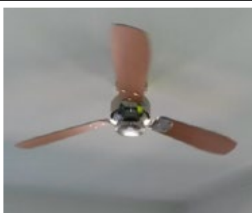
Figure 102 : Ceiling fans are installed in every office space
