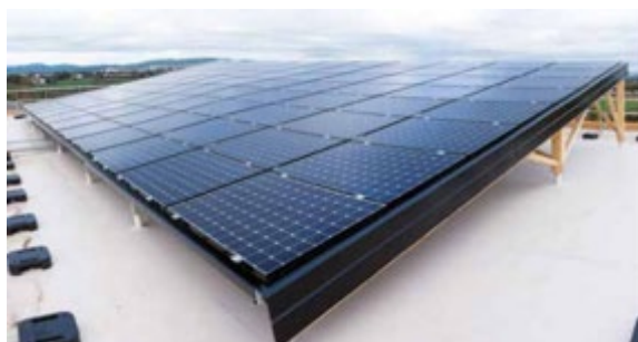
Figure 48: View of the PV panels installed on the rooftop of the building
