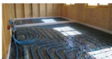
Figure 43: The building is equipped with an under-floor heating/cooling system powered by a ground source heat pump
