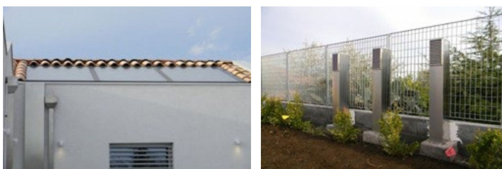
Figure 10: Pictures of installed systems (on the left: thermal solar collectors, on the right: Earth to Air Heat Exchanger) [3]
