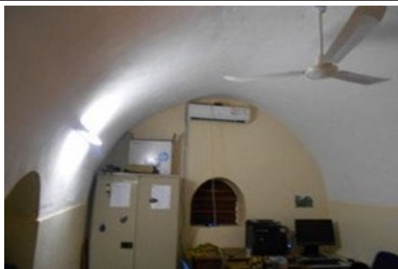
Figure 127: View of the cooling equipment of the rooms
