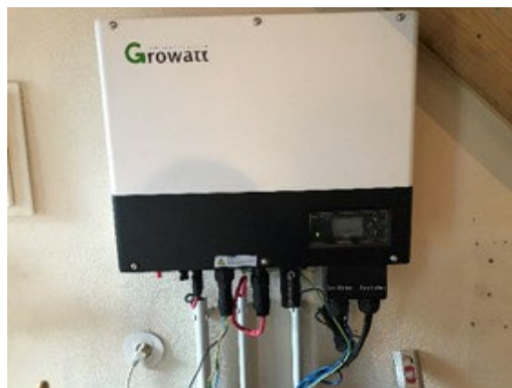
Figure 34 : View of the Growatt Hybrid inverter to PV systems, specially designed for storing current in batteries.
