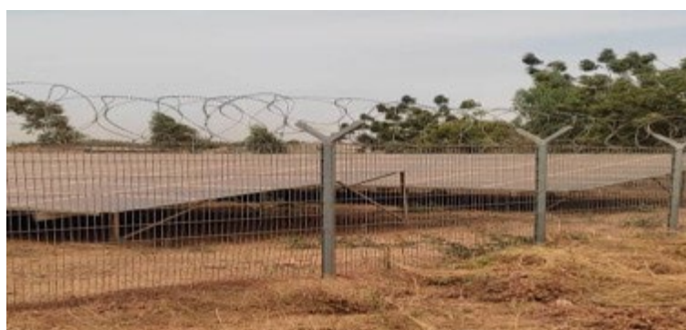
Figure 92: Ground mounted solar PV system of the BIT.
