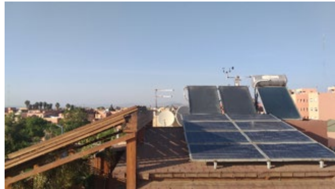
Figure 159 Solar thermal and photovoltaic panels installed on the roof of the house
