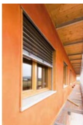
Figure 35: Motor drive external venetian blind. Type: Grinotex from Griesser.
