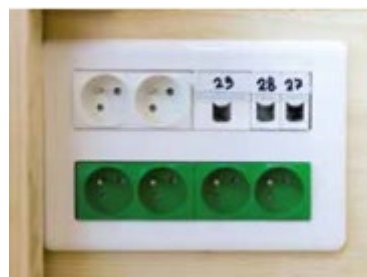
Figure 47 : Multi-socket adaptors with a power switch
