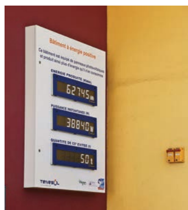
Figure 82 : PV production on the panel [2]
