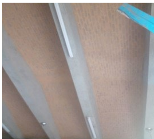
Figure 122: Interior view of the ceiling and lighting tubes.
