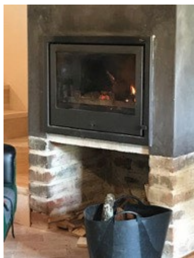
Figure 30 : View of the wood burner.
