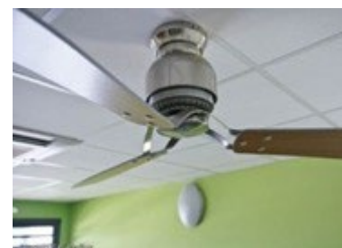
Figure 80 :Efficient ceiling fans have been installed in the classrooms.
