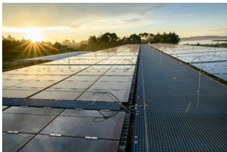
Figure 169: 3 600 m 2 of photovoltaic panels are installed on the rooftop of the building. © Emmanuel Museruka – Malaika Media
