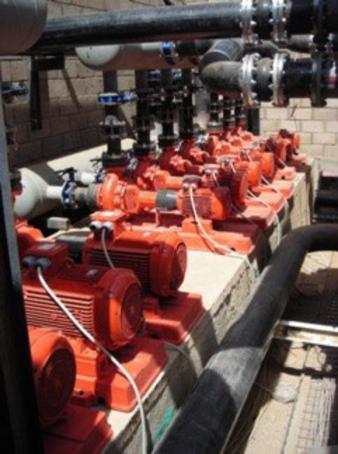
Figure 183: View of circulation pumps of chilled water [3]
