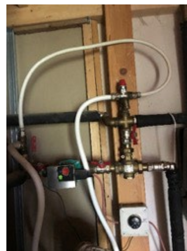
Figure 32 : View of the pipes and system that feeds the heated pavement and the hot water domestic grid.
