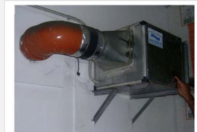
Figure 3: Point where the air from the earth tube is introduced in the building [4]
