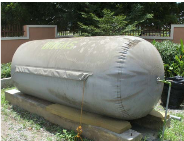
Fig. 6.4-16 – Above ground plastic inflatable gasholder
