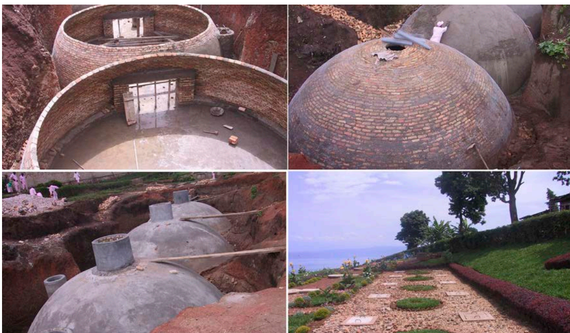
Fig. 5.2-5 – Digesters construction stages - Sources: G. P.Nembrini, A. Kimaro, Using Biogas Plants for Treatment of Urban Community Wastes to Supply Energy and Improve Sanitation , presented at the Expert Group Meeting on "Energy Access for the Urban Poor", December 2006, Nairobi
