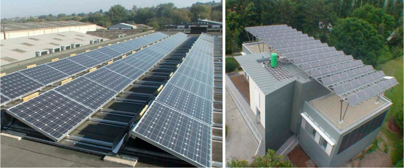
6.1-2 – PV on flat roof
