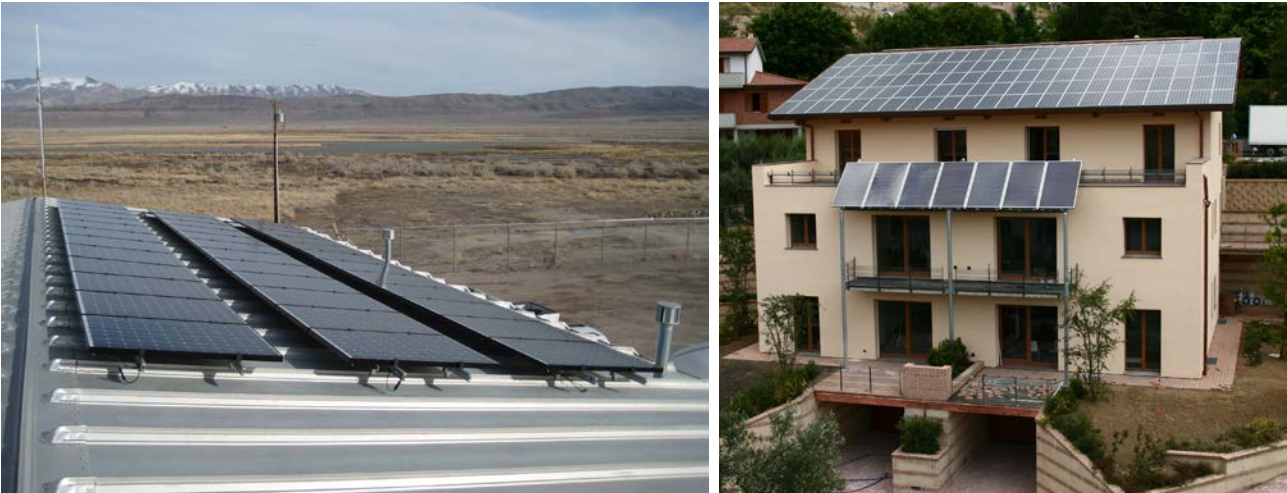
Fig. 6.1-3 – PV on pitched roof (Photo credit (left): USFWS Pacific Southwest Region - http://www.flickr.com/ )
