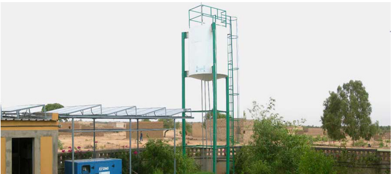
Photovoltaic and water storage system © FAREstudio
