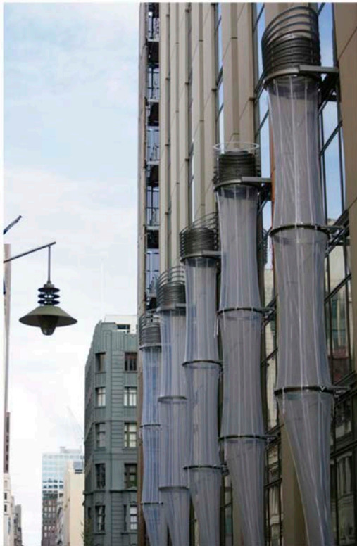
Fig. 3.8-6 – Council House 2 Cooling towers
