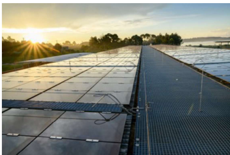
Figure 168: 3 600 m 2 of photovoltaic panels are installed on the rooftop of the building. © Emmanuel Museruka – Malaika Media
