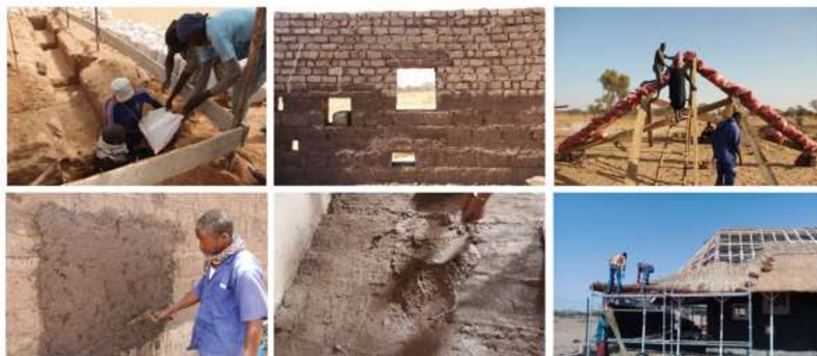
Figure 152 : Construction materials. Top, from left to right: bonded sandbags foundations, mudbrick walls, wooden plank truss. Bottom, from left to right: earth plaster, earth floor and Typha thatched roof.
