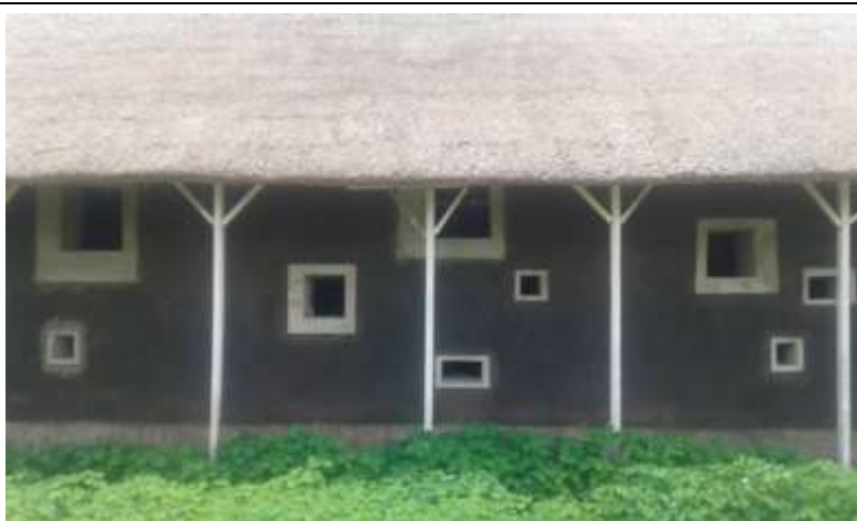
Figure 153 : Exterior view of the East façade of the classroom during the rainy season.
