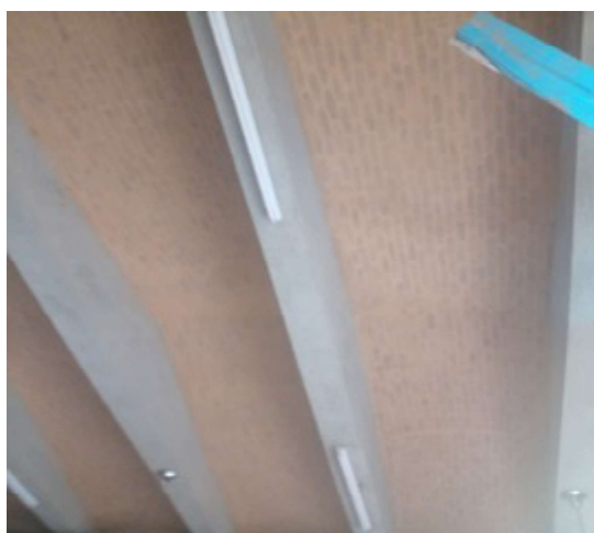
Figure 121: Interior view of the ceiling and lighting tubes.
