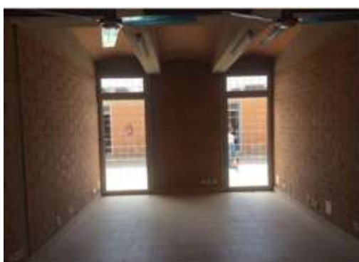
Figure 115: Interior view of the rooms equipped with ceiling fans and fluorescent tubes.
