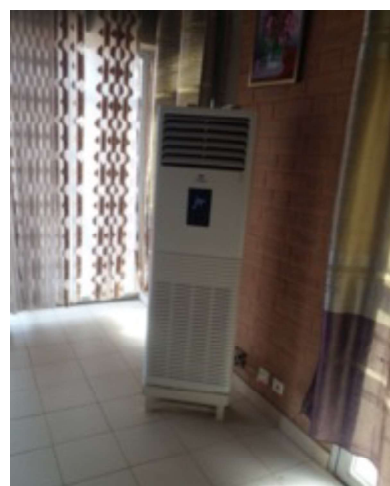
Figure 122 : Floor standing air conditioner have been installed in some rooms.
