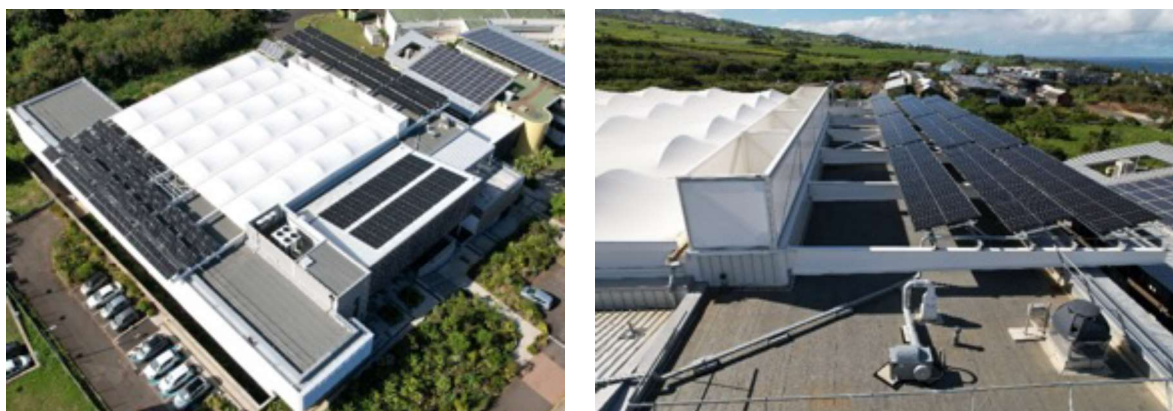
Figure 65: Solar thermal and PV panels have been installed on the rooftop of the building.
