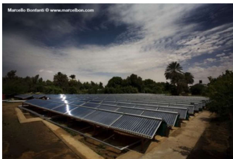
Figure 185: A solar farm of 1000 m 2 powers the water-heating system. [3]
