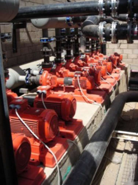
Figure 183: View of circulation pumps of chilled water [3]
