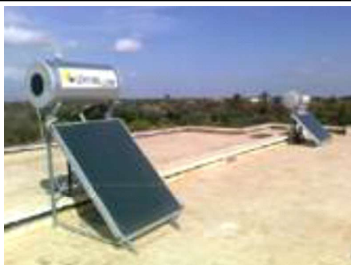
Figure 171: Solar water heaters installed on the rooftop of the Dar Amys Villa.
