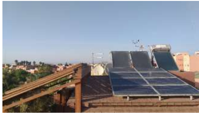
Figure 159 Solar thermal and photovoltaic panels installed on the roof of the house
