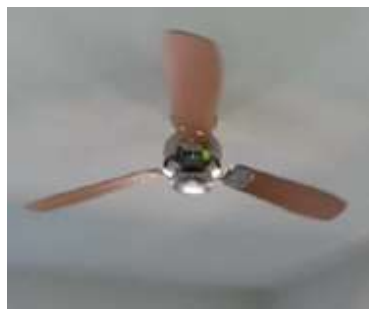
Figure 102 : Ceiling fans are installed in every office space
