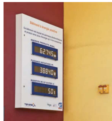
Figure 82 : PV production on the panel [2]
