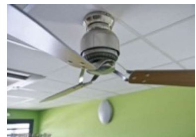
Figure 80 : Efficient ceiling fans have been installed in the classrooms.
