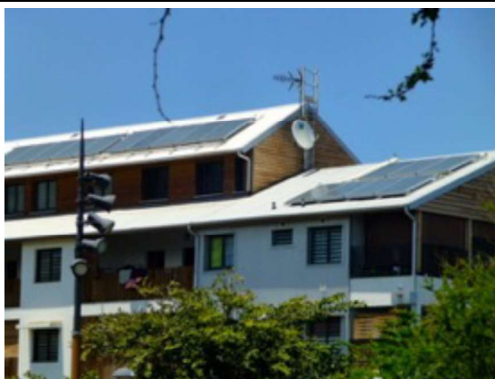
Figure 67 Solar thermal solar panels are installed on the rooftop of the building for the production of hot water
