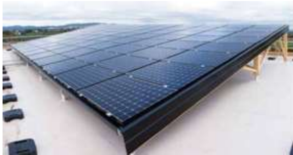
Figure 48: View of the PV panels installed on the rooftop of the building
