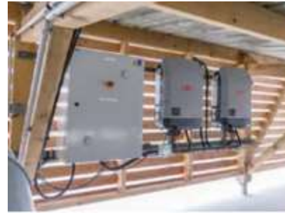
Figure 49: Solar inverter and sensors of the PV system
