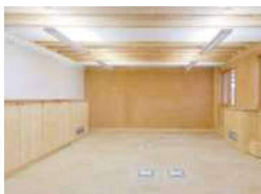
Figure 46 : Lighting of the training room with presence sensors and daylight linked dimming systems
