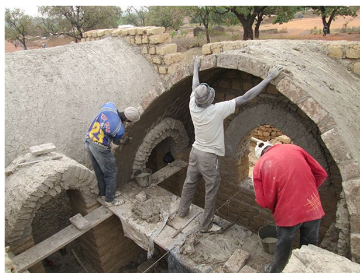
Figure 16: NV Building site of the Artisanal Production Unit in Niéna (Mali) / Source: AVN
