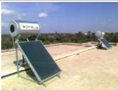
Figure 164: Solar water heaters installed on the rooftop of the Dar Amys Villa.
