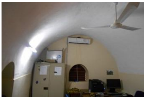
Figure 120: View of the cooling equipment of the rooms
