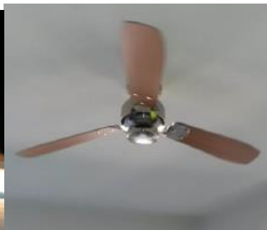
Figure 99 : Ceiling fans are installed in every office space
