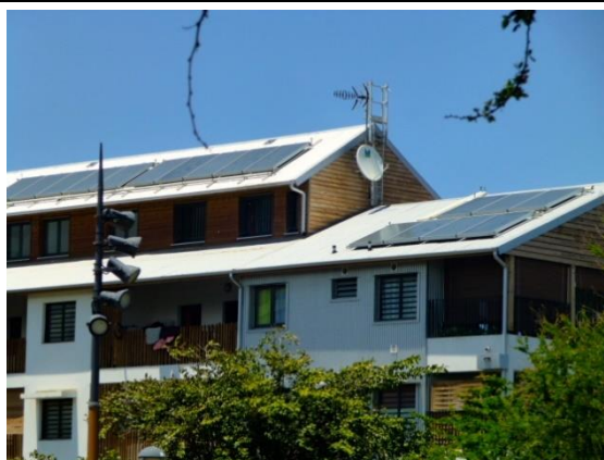
Figure 61 Solar thermal solar panels are installed on the rooftop of the building for the production of hot water
