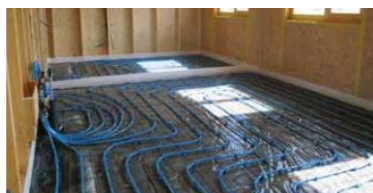
Figure 42: The building is equipped with an under-floor heating/cooling system powered by a ground source heat pump
