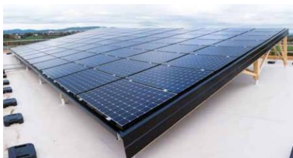
Figure 47: View of the PV panels installed on the rooftop of the building
