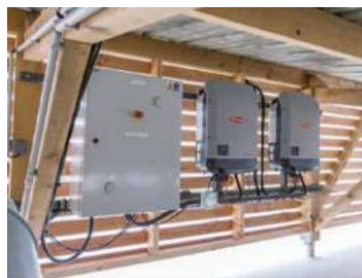
Figure 48: Solar inverter and sensors of the PV system
